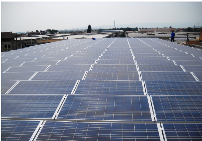
Applause for long-term thinking: Installing solar panels at their production site has helped our supplier Jumbo to avoid more than 250 tonnes of CO 2 emissions.
