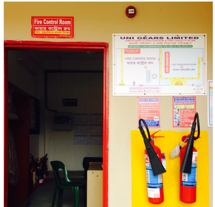
Steps factories had to take to meet the new safety code include investing in integrated fire alarm systems, fire doors and sprinkler systems.
